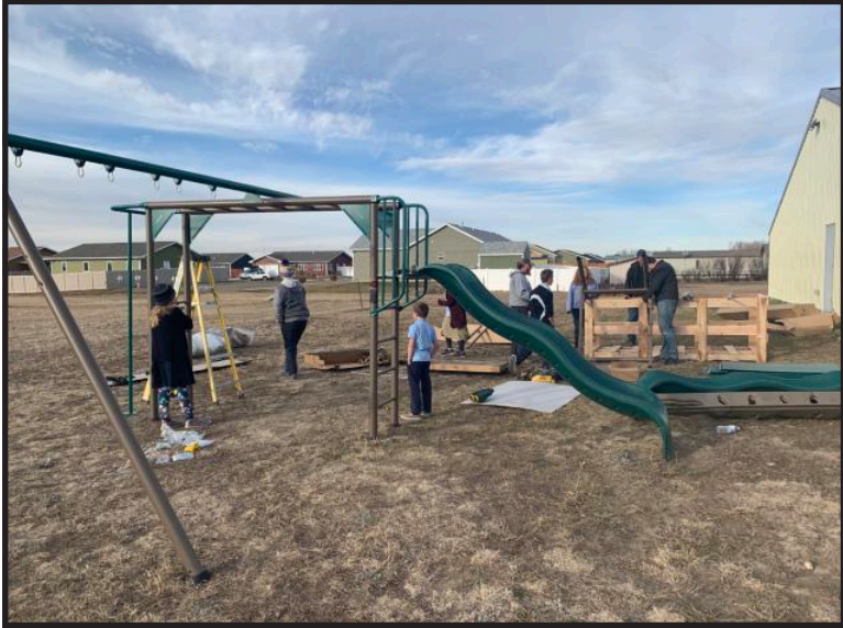
Variegated crew putting together new playground equipment Great Falls Christian Academy Christ's Church, Great Falls, MT
